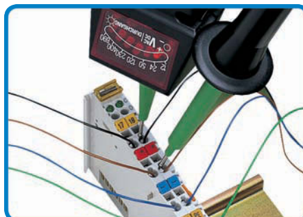
Signal tracing with wired conductors
