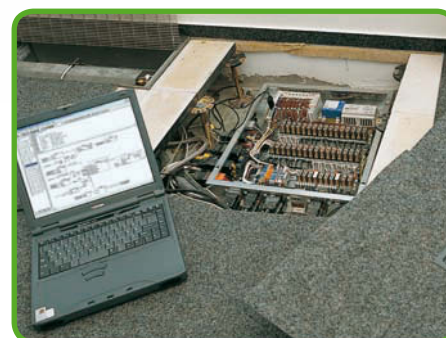
Under-floor distribution boxes
